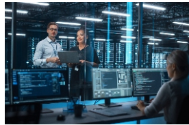
Server Room & Data Center
